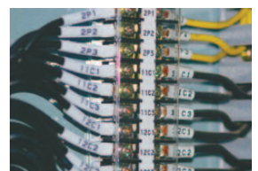
Wiring on a board
