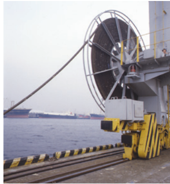
Cabtire cables for cargo cranes
