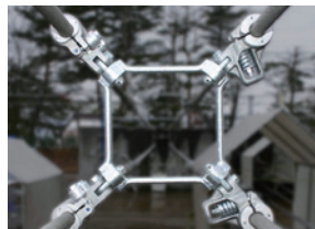
Loose spacer damper
