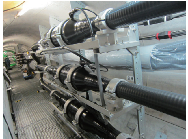
図3 駿河東清水線2 L(甲) CSJ 施工状況 View of CSJ in Suruga Higashi-Shimizu Second Line.
